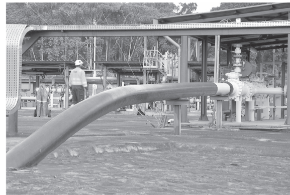
About 9 652 million cubic feet of natural gas were delivered to the Kribi power plant, corresponding to a used capacity of 149 MW
