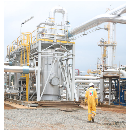
9 123.84 million cubic feet of natural gas delivered to the Kribi power plant
