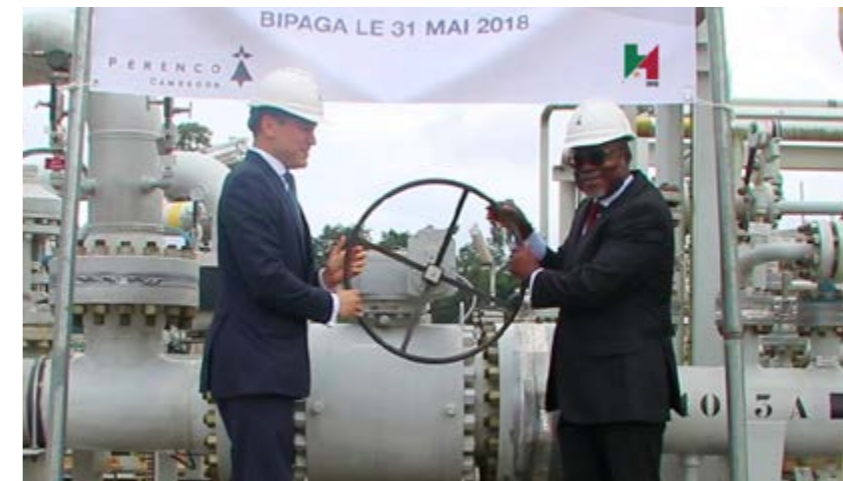
Symbolic opening of the gas delivery valve to the floating plant by Mr. Perodo and Mr. Bayiha
